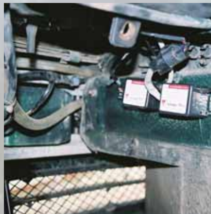
Control and igniter units (see text) are located inside the front wings – an area that's kept clean and dry by the plastic wheelarch liners. Photo above shows the view under the left-hand wing
